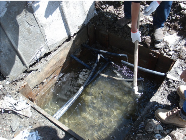
Figure 3: Upper spring source ( S_2 ) has 4 different intake pipes with a total discharge of 63.9 liters per minute.
